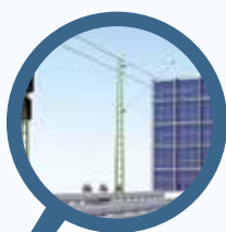
Cables for catenary
